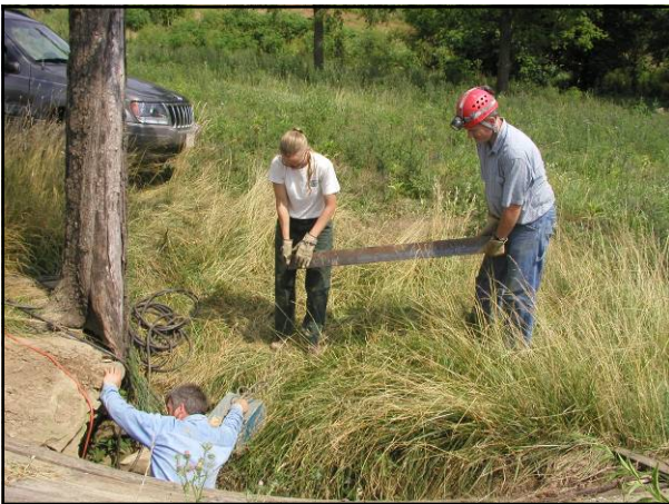
Carrying steel girders for construction of the cave gate. Photo courtesy of USFWS.
